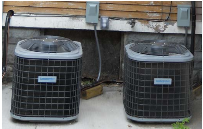
Proper grade placed A/C units with direct line installation
