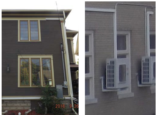
Improper installation of exterior equipment and lines can have a detrimental impact on the character of a structure.
