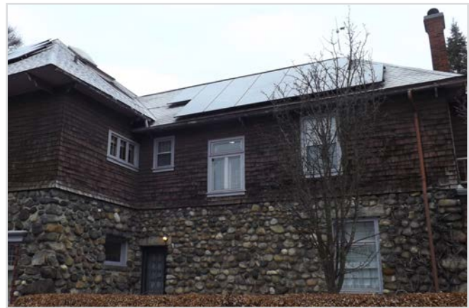
An approved Roof Mounted Solar installation located at rear
